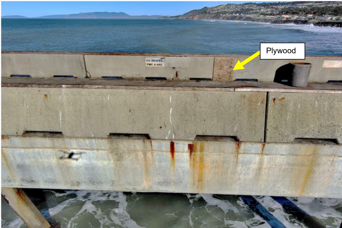
Figure 3.1 Plywood over spalling damage on handrail.
