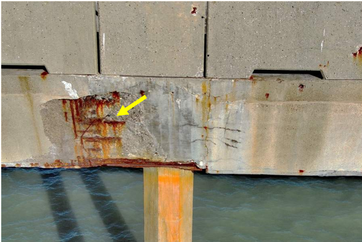
Figure 3.3 Damaged Bent O Cap, View to South.
