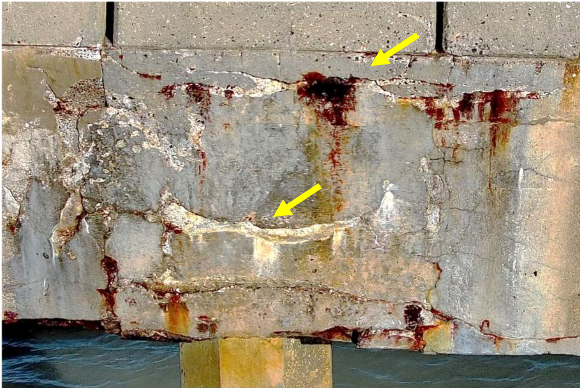
Figure 3.2 Damage at Bent L Caps, View to South.
