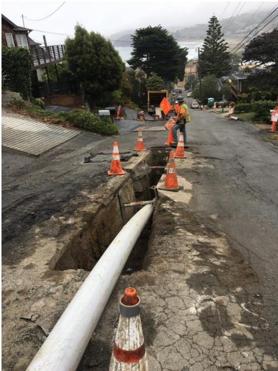
An example of the work that was done as part of the Pedro Point Sewer Rehabilitation Project
